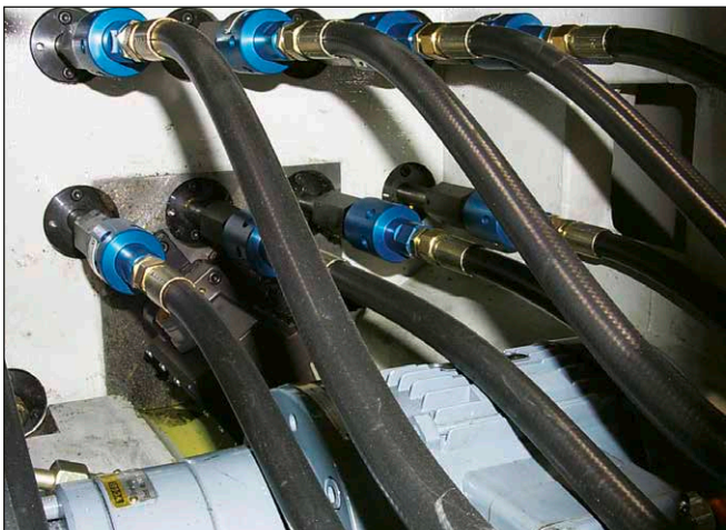
Deublin 1116 Bearing-Supported Unions on Automotive Transfer Line.
